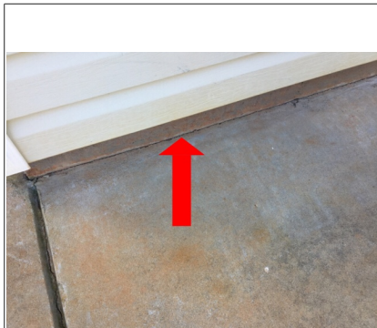
Recommend sealing where patio meets house slab. Due to slight settling, a small gap has been created between slab & patio.
