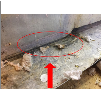
Fresh water found in emergency condensate pan at time of inspection. Recommend licensed HVAC technician evaluate & service attic unit for left side of home.
