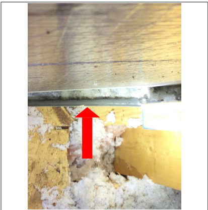
On same unit in attic for left side of home. Wet insulation was noted in emergency condensate pan behind unit. Recommend repair.
